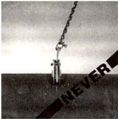
Photograph D (Typical) Excessive sideloading.
